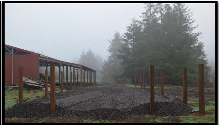
Runoff Management: Gutters, Downspouts, Drainpipe, and Heavy Use Area.
