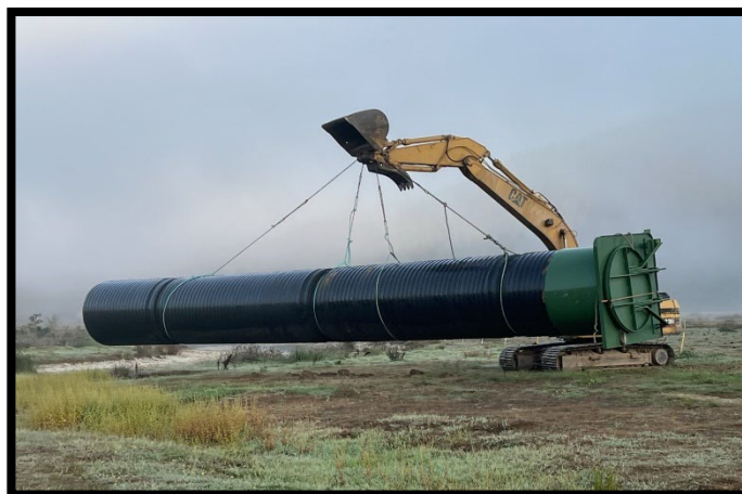
September 2023 – One of the tide gates & culverts being moved to the installation location.
