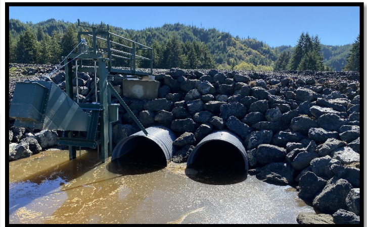
Interior view of MTR System with walkway installed on the left, and tide gate culverts installed on right.
